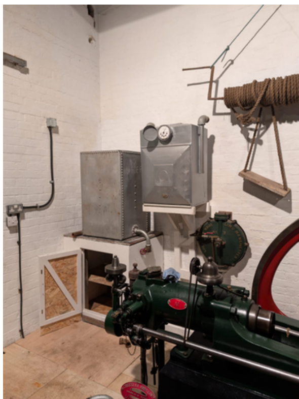
The new cooling tank for the gas engine.
